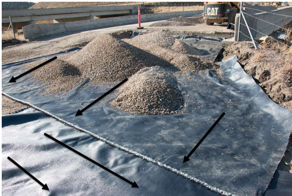
Image 5 - Bridge Approach, Routing Water Away from Structure.
