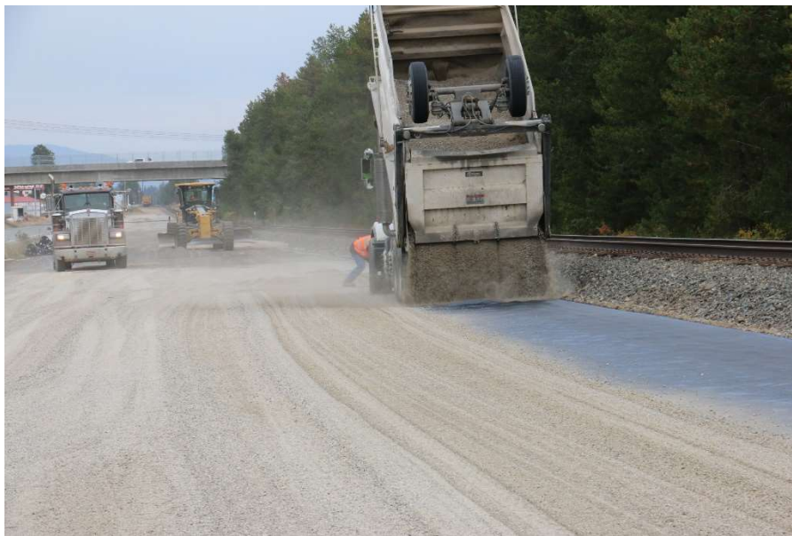
Photo 17. Gate Set to Spread 1" (25 mm) Lift Allowing a Full Spread Over One Roll.
