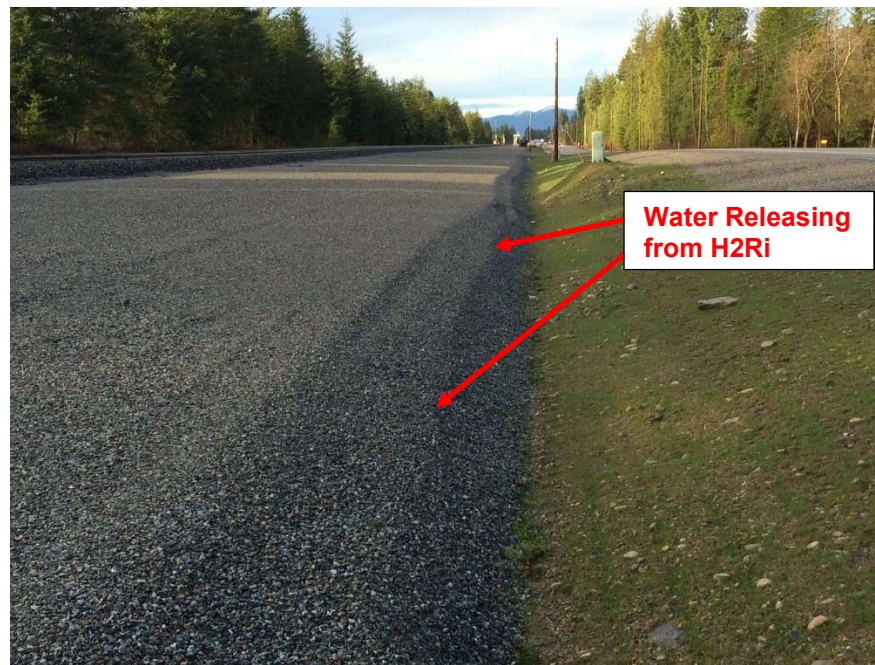
Image 10 - Water Wicking with Edge Termination
