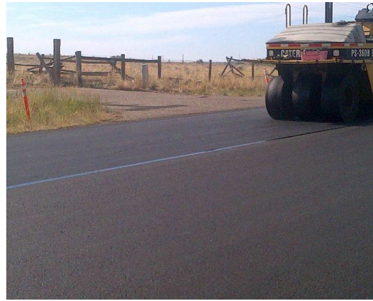
Image 4: A pneumatic tire roller is recommended to bond the GlasPave mat to the tack coat in certain scenarios.
