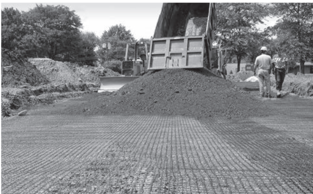
End dumping aggregate fill on top of Tensor Geogrid over soft subgrade.
